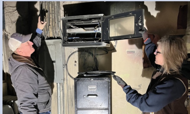
Camp directors Ray Queen and Julie Minnick examine fire damages at Camp Blue Ridge's Town Hall.
