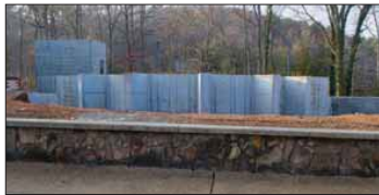
Southern's new nursing building is being constructed in the old Jones Hall parking lot.
