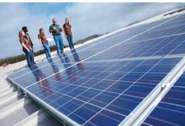
Dave Allemand, associate director of Plant Services, goes over the details of the solar panel installation with visiting SIFE students.
