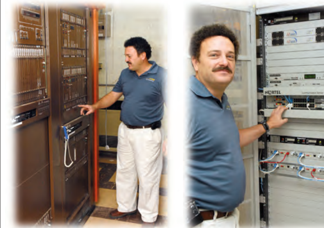
The old communications system is now being replaced with the latest technology that consolidates and entire room of switchers into one small electronic computer tower.
