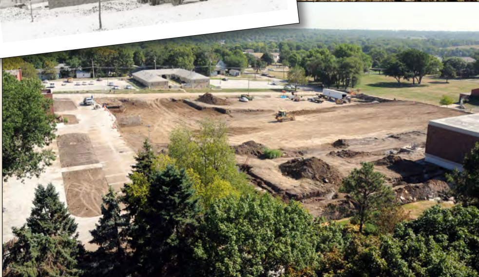
Above: A newly completed circle drive behind Rees Hall will be open in time for the women to move into the dorm this fall (June 12, 2012). Left: The building site is prepared, and workers will begin pouring footings in mid-August (July 19, 2012). Far left: Workmen continue to brick the walls of Jorgensen Hall, even through winter snows.
