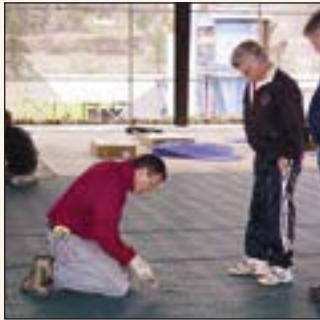
The resilient flooring that has been installed in the Falk Sport Court will make it safer for the students. Left to right: Mike Taylor, Sport Court Representative; Bill Coach; Randy Bovee, Principal
