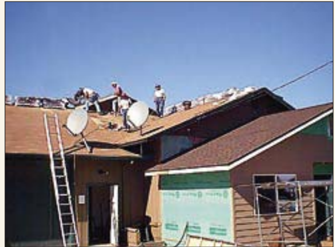
Maranatha volunteers help with a building expansion and remodeling project at the Better Life Television station in Grants Pass.
