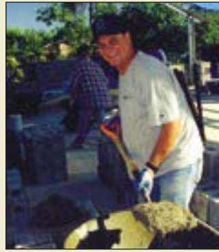
Al Griffone from Arlington, Wash., keeps the block layers supplied with mortar.
