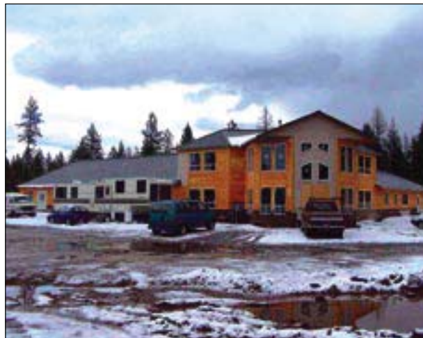
A new church is being built just off Highway 95 in Hayden Lake.
