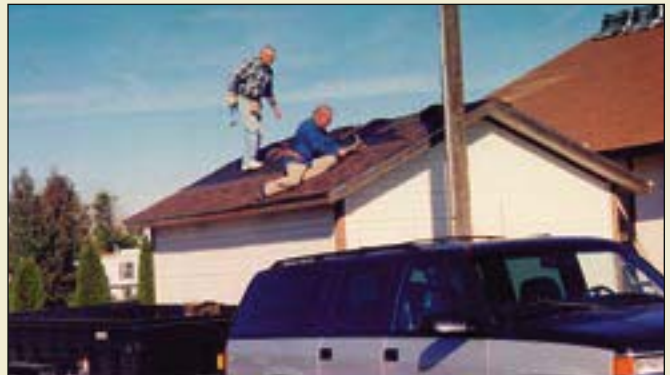
Ted Lutts and Joel Stahl install new roofing on the well house.
