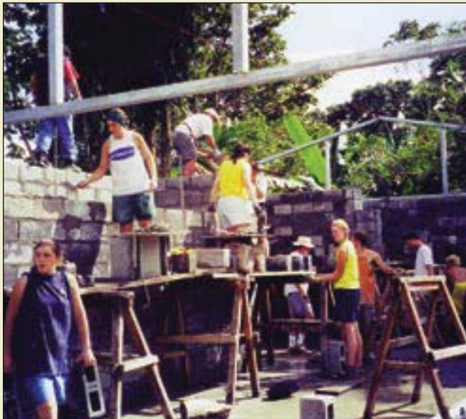
Work on the block walls of the classroom advances as PSAA students enjoy a break in the torrential rains common during their mission trip to Baatan, Costa Rica.
