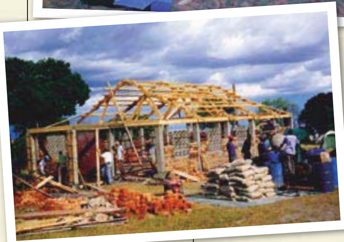
Cascade Christian Academy students participated in the construction of a church during a recent mission trip to Kenya.
