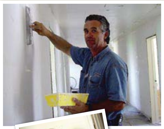
Jeff Wade of Precision Builders applies texture to the walls during the renovation of the girls’ dorm.
