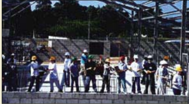
The quickest way to get the cement blocks from the outside to the inside was via "the block brigade."
