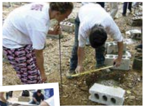
Tricia Kimbrough, AAA senior, and Keith Hallam, AAA principal, work together building at the youth camp amphitheater project in Puerto Rico.
