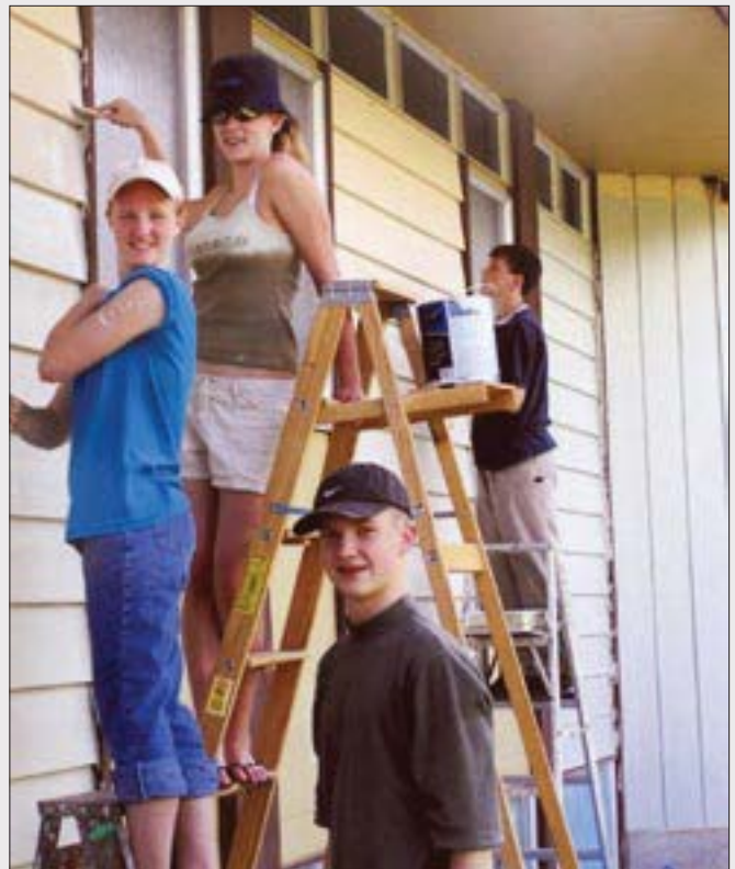
Kids from Spokane Valley Adventist School helped to paint the Brewster Church in June.
