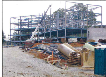
This construction project in Tennessee is one of the many projects that Mark Black manages across the nation.
