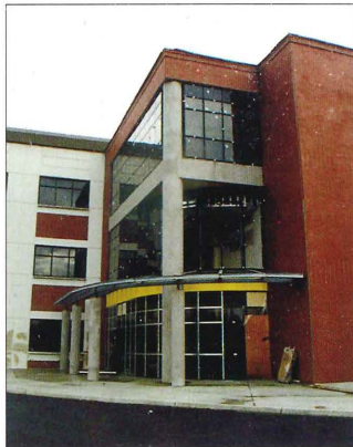
The walls are up at Gresham Station, where Adventist Medical Center is building a high-tech outpatient imaging center.
