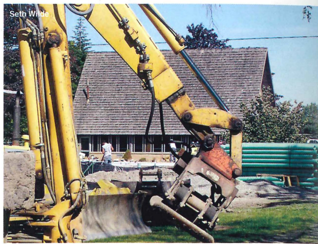
Foundations for the new girls' dorm at AAA have been poured and construction is continuing.
