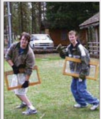
Brothers Micheal and Daniel Jeffery "carefully" salvage windows from a building the group tore down.
