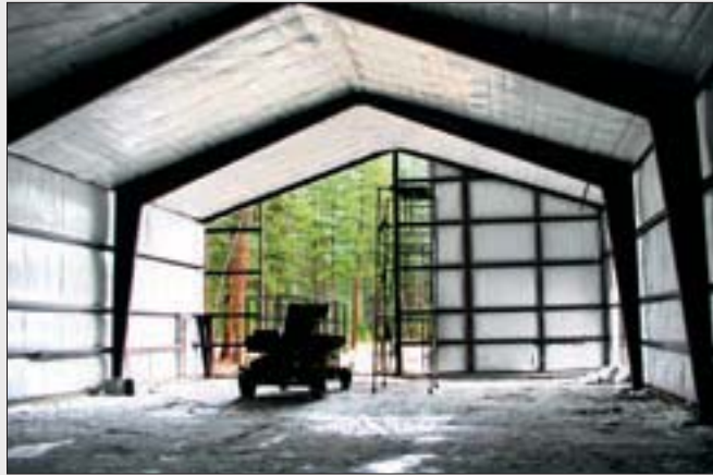
A neighboring contractor saw the Libby School's gym being built and offered the use of his scissor lift to help install the roof.
