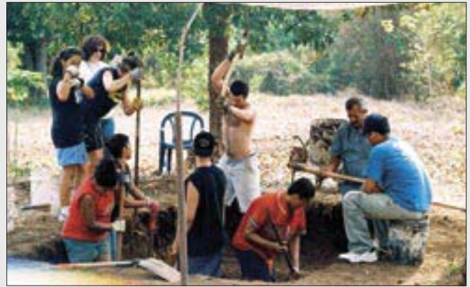
Digging a septic tank by hand was a challenging task for teens on the Oregon Conference mission trip.
