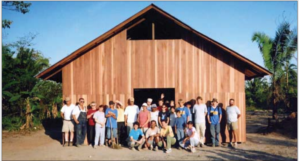
Team members worked in 105-degree heat to put the mahogany siding on the church.
