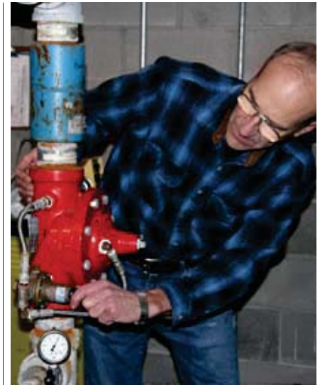
Gary Bartholomew installs and services pump systems in Spokane, Washington. He was inspired to use his knowledge to drill wells and install a water system for the ICC school and orphanage in Guatemala.
