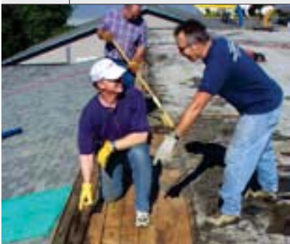
Members in Coeur d'Alene work to put a new pitched roof on the Lake City Junior Academy gym.
