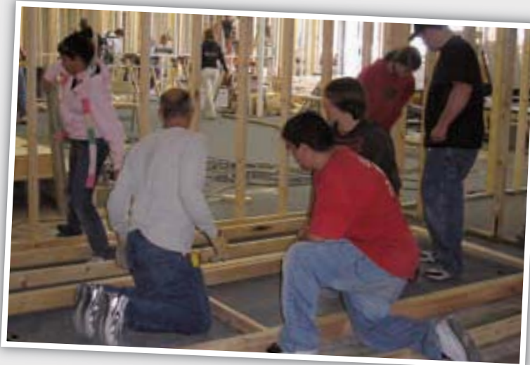
One of the Teen Mission Adventure projects was framing the interior walls of the new Brewster Hispanic Church.
