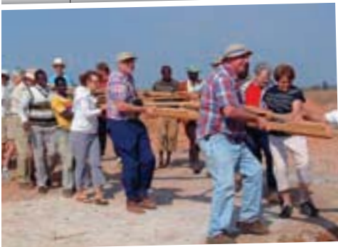
Most of the team, including doctors, nurses and pastors, helped put the roof trusses in place for a new three-room school building.
