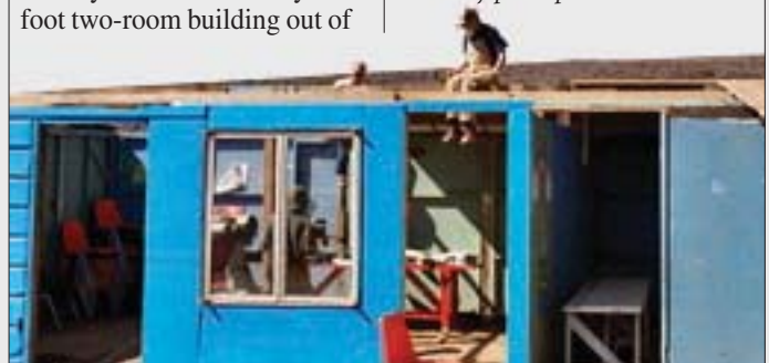
The Hermiston crew built a two-room building of scrap lumber materials for a local pastor.
