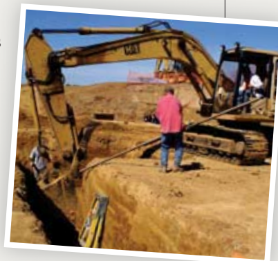
September 6, 2005—Earth-moving equipment and excavators dig deep into the clay earth for the basement.
