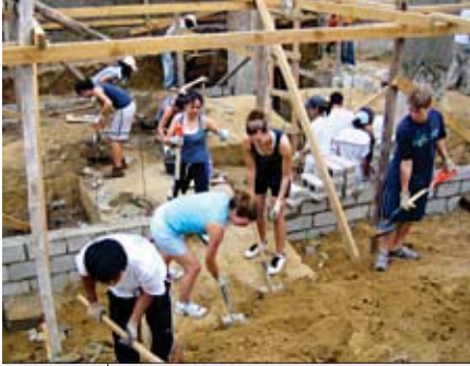
PSAA students level dirt inside the walls of the Dulce de Luna School in preparation for the concrete floor.
