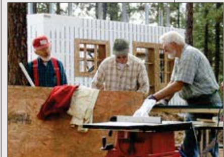
Ken Carr, Birney Brown and Darrel Hall puzzle out a piece to be installed in one of the guest cabins.
