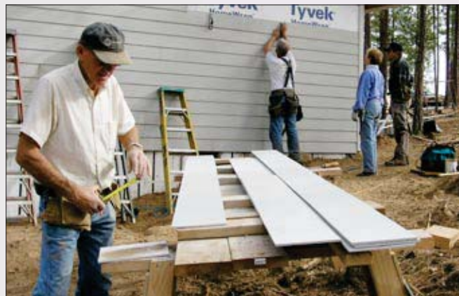
Maranatha volunteers make quick work of installing the siding on the guest cabin.
