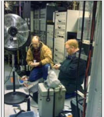
Bill Whitt, Better Life engineer, installs an Astoria transmitter.
