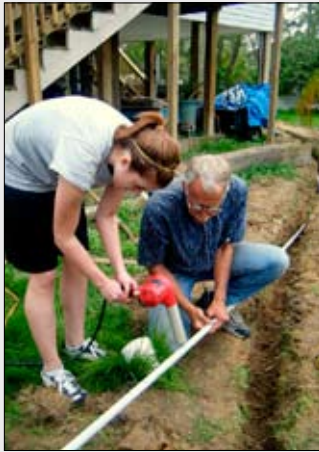
Todd Johnson, HHFM leader, teaches Ellie Evans to heat and bend a PVC electrical pipe.
