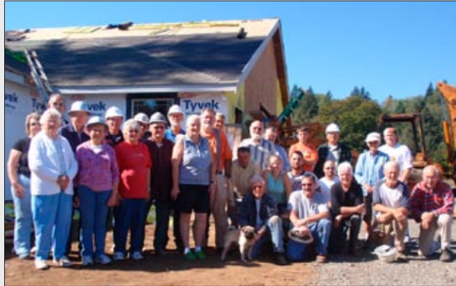
Twenty-five to 30 volunteers from Maranatha International came to Yacolt, Wash., the last part of September to build a church.
