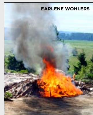
Lewis County Adventist School in Chehalis, Wash., members work with the local fire department to burn down their 57-year-old school facility to make way for a new school facility.
