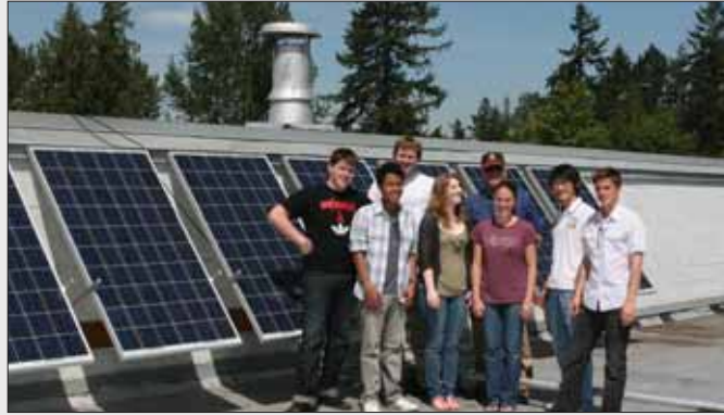
Students enrolled in engineering classes at Auburn Adventist Academy, install eight solar panels to help reduce the carbon footprint of the campus.
