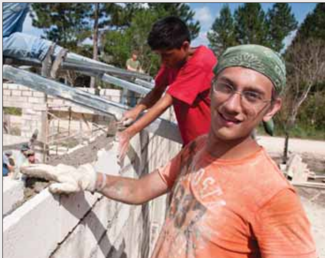
Home-school student Skyler Bushnell adds concrete inside the top layer of blocks for a new church in Guatemala.
