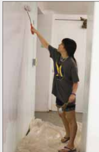
Christine Kim is part of the paint crew during the mission to renovate Hawaii's Kahili Mountain Park.
