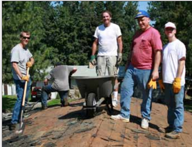
Spokane-area church members help remove shingles from the roof of a community member needing help.
