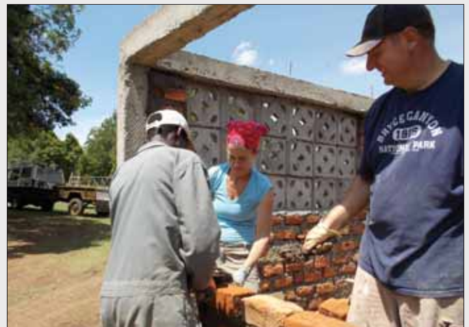
Shelby Vercio and Greg Allen finish the last wall of the project.
