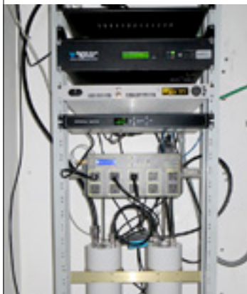
The equipment rack holds needed equipment for the radio station.
