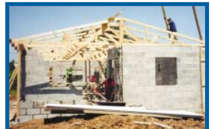
Duane Carlisle works on the roof of the house that was constructed for a needy mother with four children.
