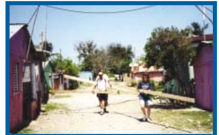
Bob and DeLynn Shepherd and Allen Smith carry supplies to the house building site.
