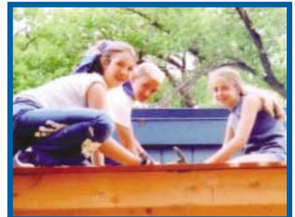
From left: Kimberly Cooper, Adam Cain, and Tori Steely repair a roof at the Chinle Mission School.
