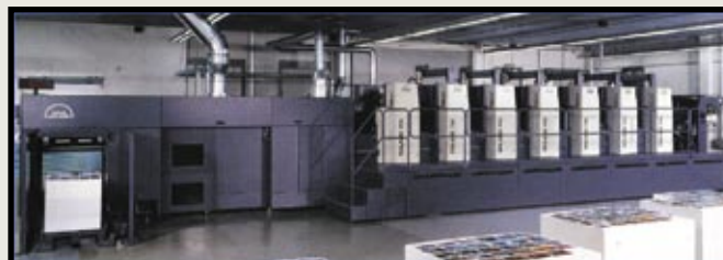
New six-color sheet-fed press now being installed at Pacific Press®
