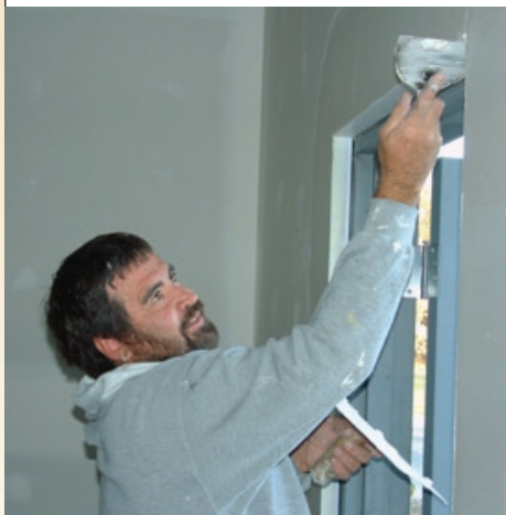
Steve Martin puts finishing touches on the drywall in one room of the Little Oaks Preschool.
