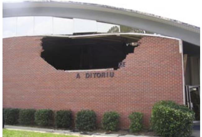
The hurricane left a hole in the academy’s gymnasium.
