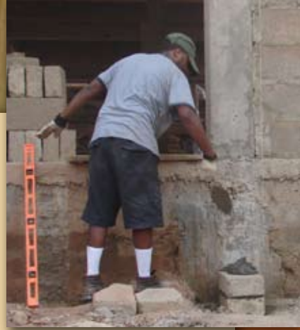
Isaac Palmer cemented blocks in a portion of the wall for the girls’ dormitory. Jim Today, Hector Ramos, Jim Redfield, and Linda Main were also on the AMH construction crew.
