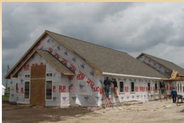
Storm clouds loomed overhead as volunteers struggled to make the new church weather tight before the rain came.
