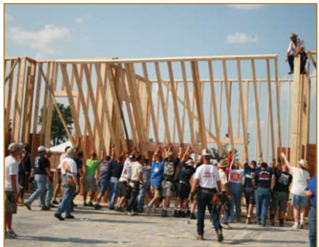
A wall was erected at Baker's Chapel in DeGonia Springs, Indiana. Hundreds of people from around the country came to help rebuild the church destroyed by a tornado. Debbie Burns was there to lend a helping hand.
