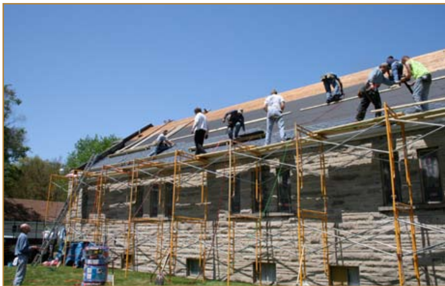
Working side by side all day, the work crews from the Cicero and Terre Haute Churches were able to enhance God's house in Terre Haute.
