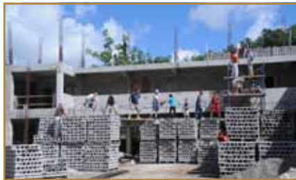
Betty and Don Schrenkel, and Darla Short, Wright Church members, shouldered the responsibility of organization of the construction progress.
