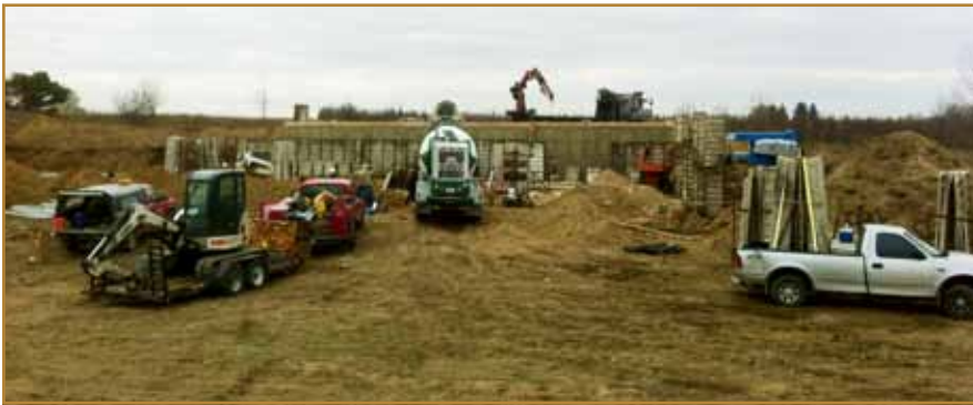
Construction has begun for the new Lake Union Conference headquarters. The basement walls, footings and elevator base have been poured.
