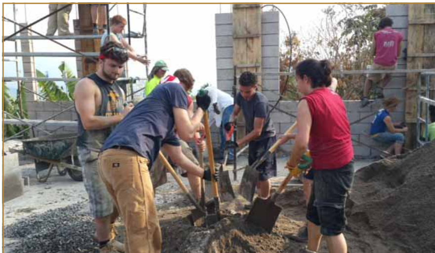
A foundation established by Paul Hufnagel helps fund mission trip expenses for Indiana Academy students. Here students prepare cement to lay blocks for a new church structure.
