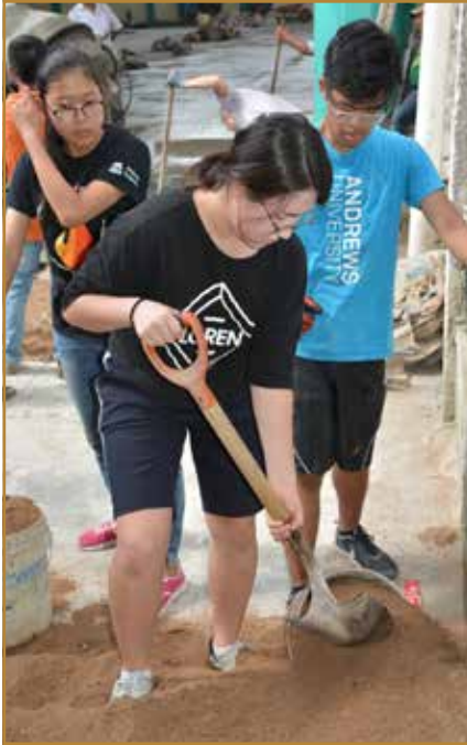
They mixed the concrete and built the floor for the school's gymnasium.
