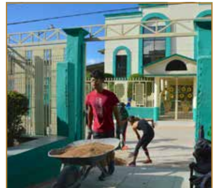
While the majority of the students had never done construction work at all, they joyfully put on their work gloves and went to work shoveling and hauling tons of gravel by wheelbarrow and buckets.
