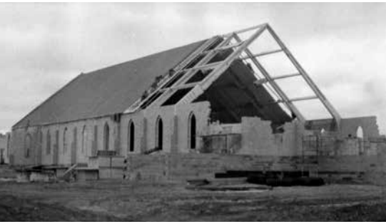
▲ Pioneer Memorial Church construction began with the groundbreaking ceremony in 1957. This photo was taken in 1958.
