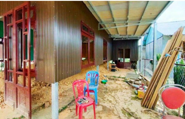
Da Chais Church, which began at the house of Chil Phi Crieu Ha Vung in 1990, has been constructing the church building, but currently funds are insufficient.
