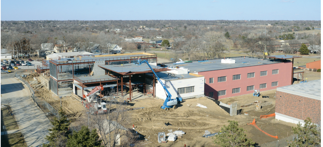
The new science and mathematics complex at Union College is rapidly taking shape even as the capital campaign to fund the project also nears completion. The Division of Science and Mathematics plans to start holding classes in the new building in January of 2014. (Photo taken March 2013)
