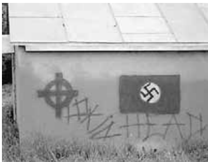
A building at the Adventist seminary in Zaokski, Russia, that has been vandalised.
