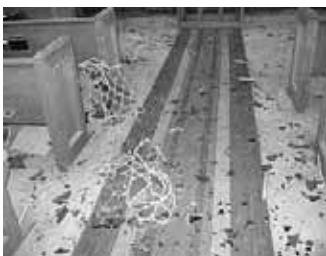
Shattered glass from the bomb blast litters the aisle of the church.
