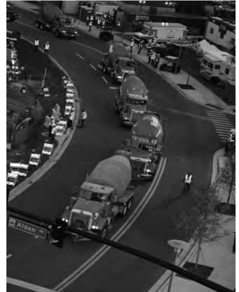
Trucks carrying loads of cement arrive for the foundation-laying at Florida Hospital.
